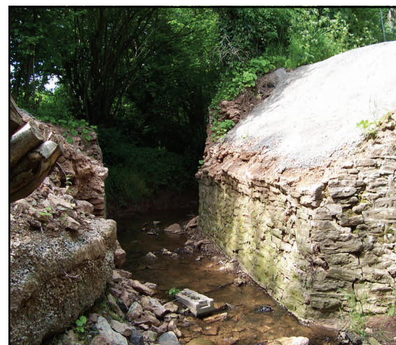
Winterburn bridge - removed due to damage
